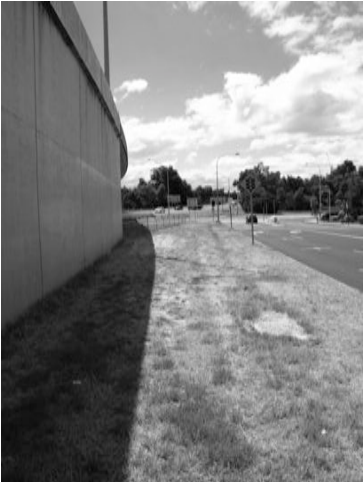
An opportunity for a landscape treatment to mitigate the visual hostility of a concrete wall.
