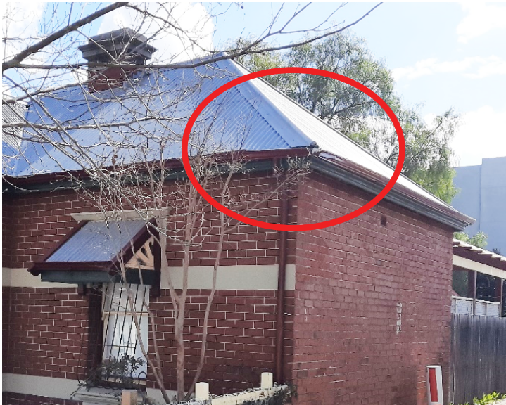
Photos: property damage at Aberdeen Street
